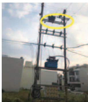
Figure 2. Metering on Proactive Repaired 200 kVA DT
