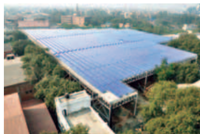
Rooftop solar is concentrated in the commercial and industrial (C&I) sector
