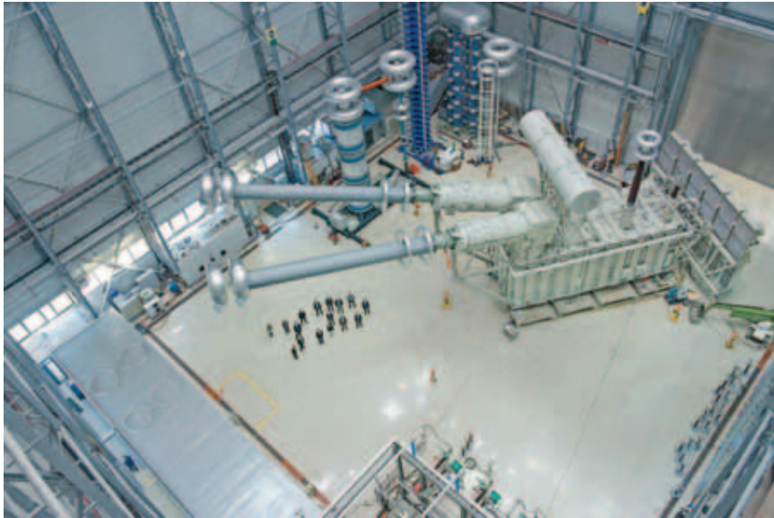
To create the high-voltage direct-current link between the Chinese cities Changji and Guquan, Siemens delivered the world's first +/- 1,100kV DC converter-transformer
